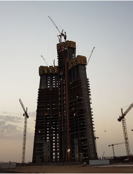
Ammar shaker, Jeddah Tower being built in northern Jeddah, Saudi Arabia. Building progress as of 13-Jul-2016 ( https://commons.wikimedia.org/wiki/File:Jeddah_Tower_Building_Progress_as_of_13-Jul-2016_003.jpg ), https://creativecommons.org/licenses/by-sa/4.0/legalcode
